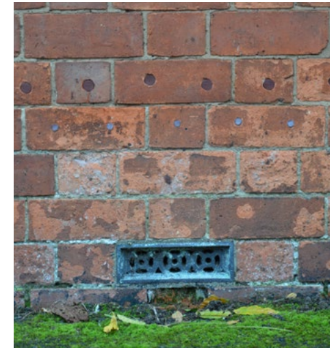
Two different attempts to resolve damp issues through inappropriate and unsympathetic methods
