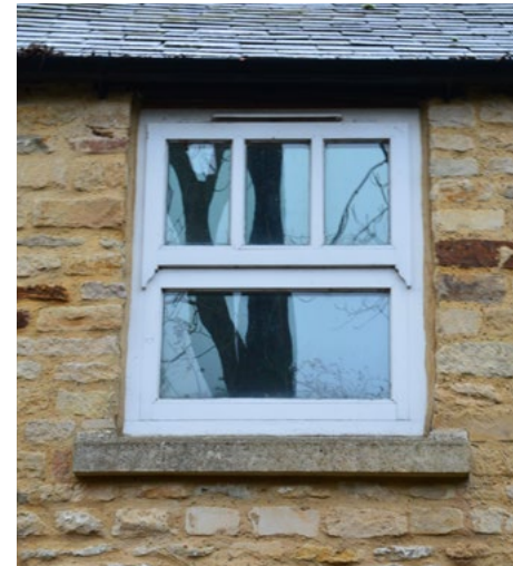
Unsympathetic UPVC window with inappropriate detailing
